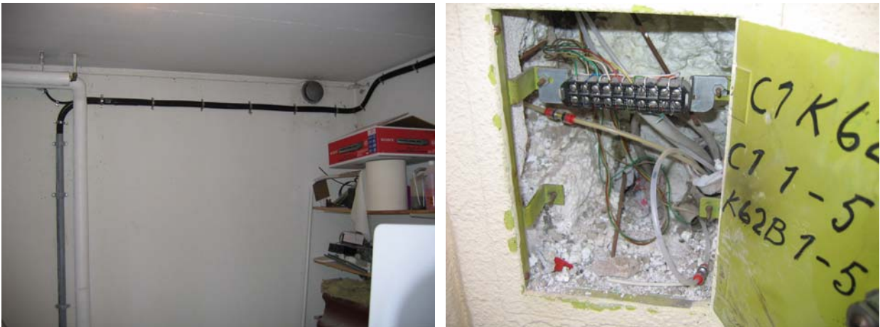
Figure 7: Bends in the microducting. Left the bundles of 4 mm microducts, 12 of them in black flexducts mounted on the walls, and right an existing wall box with lack of space.
