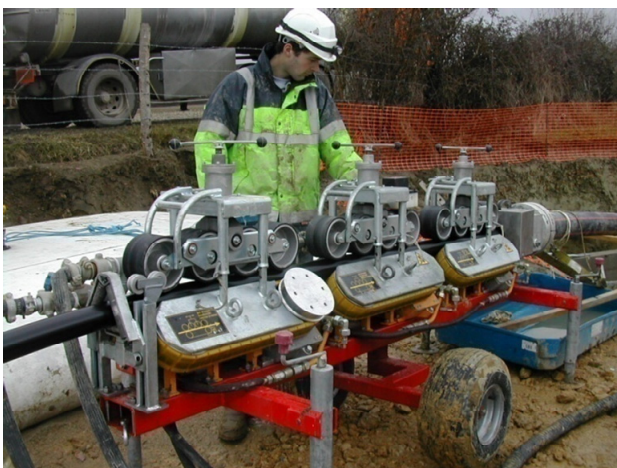
Fig. 11: WaTuCab installation of 72 mm 90 kV cable (630 mm 2 Al core) into 160/132 mm HDPE duct
