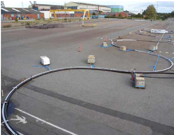
Fig. 9: Pipe windings and loops in Lindø trial
