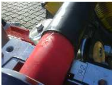
Fig. 10: Cable vulcanized joint
